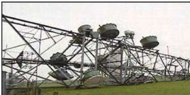
Fig 1. Cranlome Telecommunications Mast: felled in December 2002.
